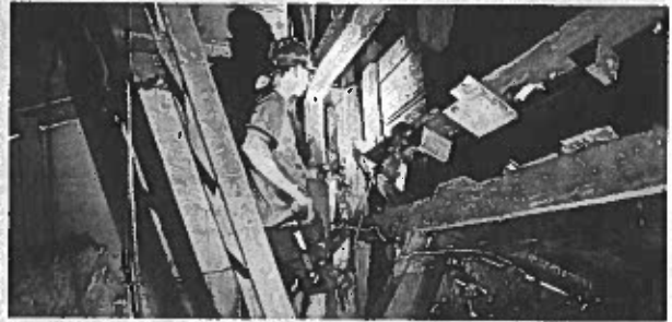
Contractor Dave Lesonik Jr. attaches four 20-foot bolts to the new bell covering inside the Little Church on the Hill. GREG WOHLFORD/ERIE TIMES-NEWS
