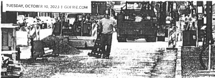
Matt Casey, 31, with XL Excavating, works in the south-bound lanes of State Street in Erie on Sept. 27. PHOTOS BY GREG WOHLFORD/ERIE TIMES-NEWS
