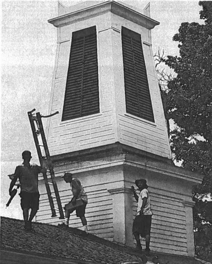
From left, contractors Dave Lesonik Jr., David Jullante and Gabe Colon clean up on Friday after attaching a new cover for the bell at the Little Church on the Hill in Elk Creek Township. GREG WOHLFORD/ERIE TIMES-NEWS
