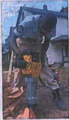
AmeriCorps National Civilian Community Corps team member Ramon Smith, 21, of Savannah, Georgia, jacks hammers a piece of concrete to clear a hole for a fence post on Friday at the corner Parade and East Fourth streets in Erie. Smith and six others from the AmeriCorps NCCOC program are in Erie for eight weeks working with the Bayfront East Side Taskforce and Our West Bayfront on neighborhood improvement projects.
