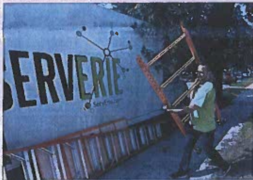
Pete Gray, tools and supplies coordinator with ServErie, loads scaffolding into a truck on Tuesday at the ServErie storage facility in Erie. Starting Thursday, volunteers from ServErie will be renovating Pfeiffer-Burleigh Elementary School and the Booker T. Washington Center. (JACK HANRAHAN PHOTO/ERIE TIMES NEWS)
