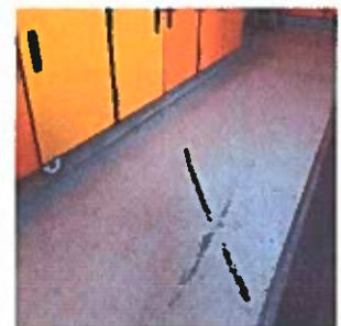
Figure 1: Cleaning of hallways, lockers and classrooms are needed.
