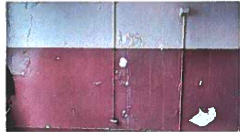
Figure 3: Previous water damage and chipping paint will be repaired and the interior of the hallways and classrooms will be repainted.
