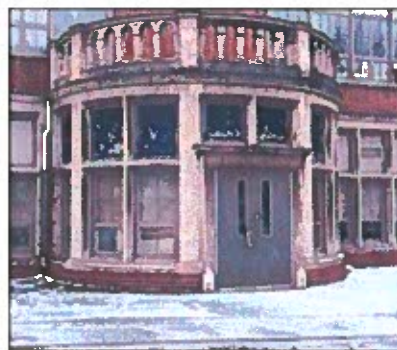
Area above doors needs painted
