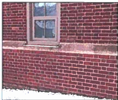
Concrete sills need power washed
