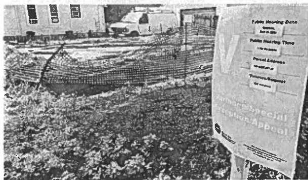
The Erie Zoning Hearing Board has approved a use variance that will allow the Sisters of St. Joseph Neighborhood Network to construct a largely underground greenhouse in the 400 block of West 19th Street, shown here on July 14.
