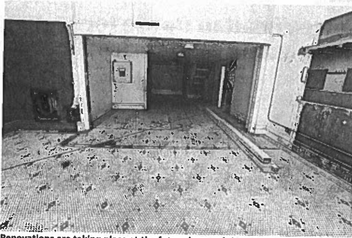
Renovations are taking place at the future home of the Purrista Cat Cafe, located inside the Erie Masonic Temple building at 32 W. Eighth St., in Erie. An original marble floor was revealed when old carpeting was removed.
